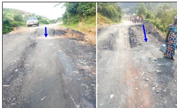
Fig 5: Subsidence and sliding of the road at Bamba-Nyamasasa
