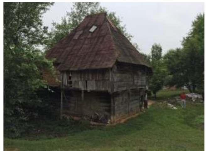
Fig 14: The Kantarevic family house in the Klupe village near Velika Kladusa. The house's current appearance
