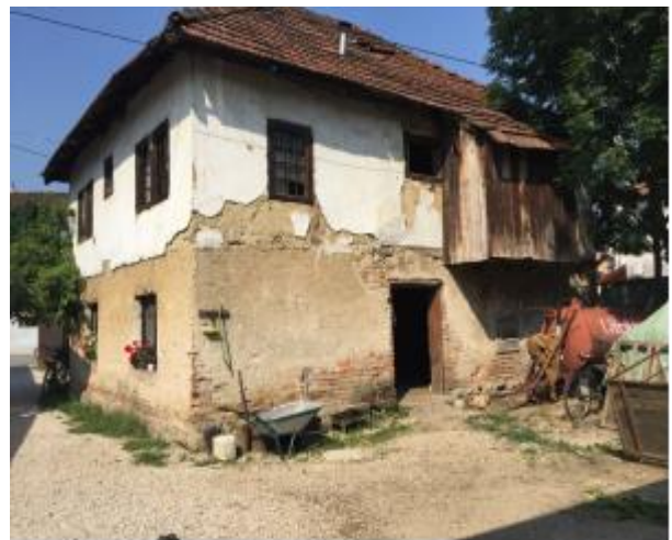
Fig 18: View of the Aganovic family house from the southwest (left) and from the east (right)
