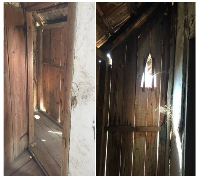
Fig 19: Toilet in the space of the 'vodnica' with access from the sofa area on the first floor
