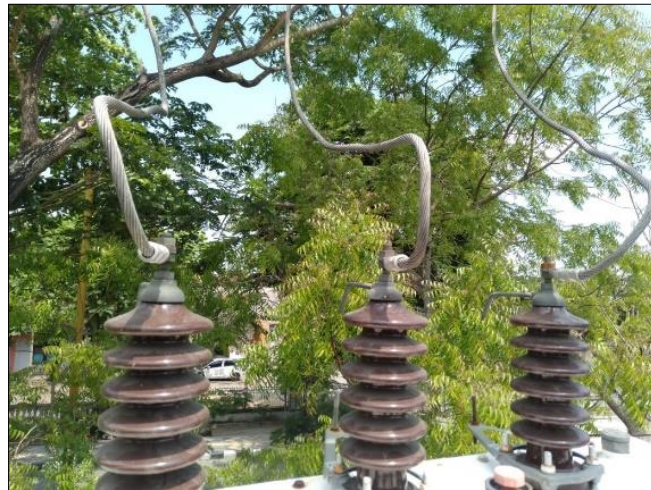
Fig 7: Visual Bushing TM Transformer
