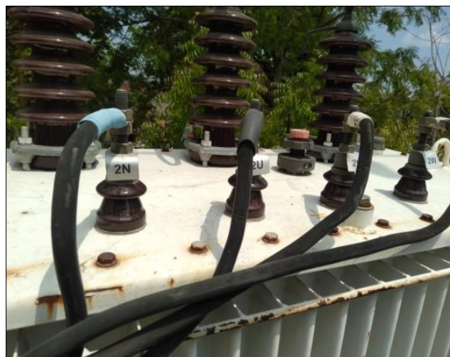
Fig 9: Visual Bushing TR Transformer
