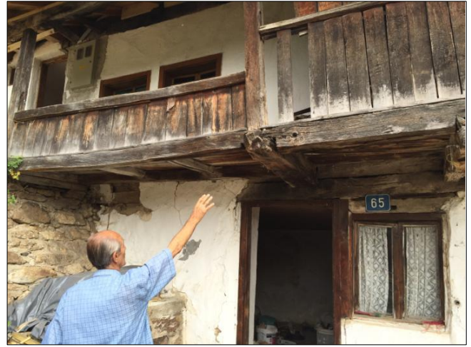
Fig 14: Place of exit of the wooden part of the staircase ground floor-first floor on the (original) divanhana and subsequent extension of the divanhana-veranda (left)
