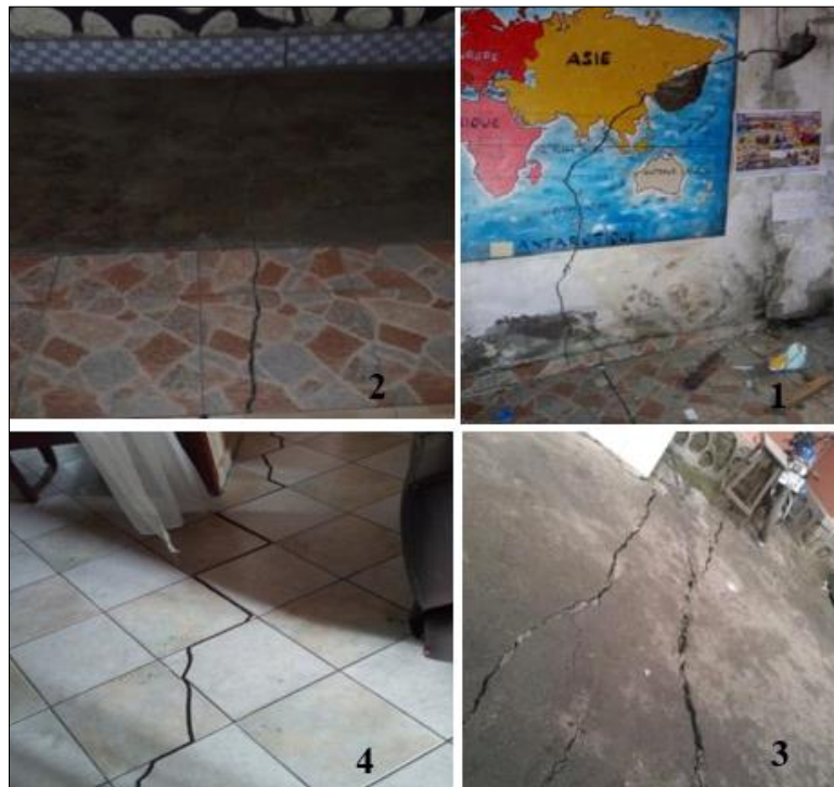
Fig 7: (3, 4) House cracks and (1, 2) Schools
