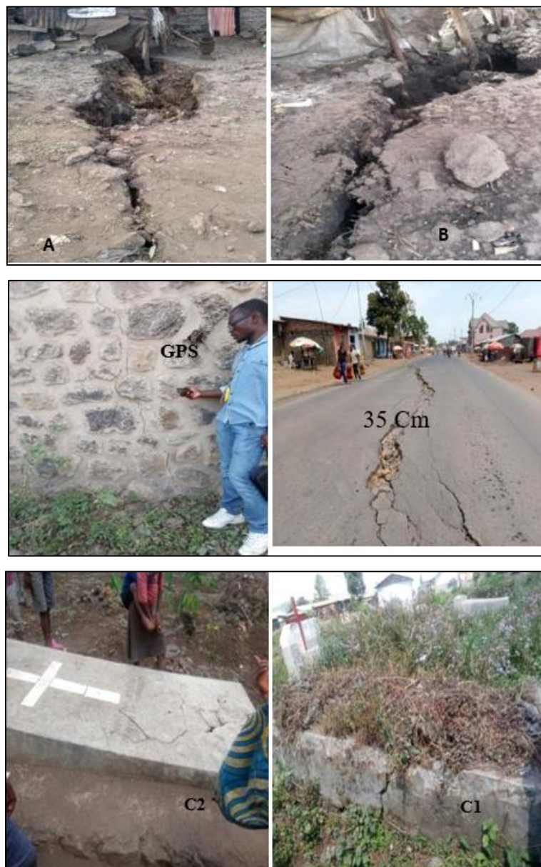
Fig 6. (a) Destruction of the wall, (b) airport road and (c 1 c 2 ) the graves of the SEP CONGO cemetery
