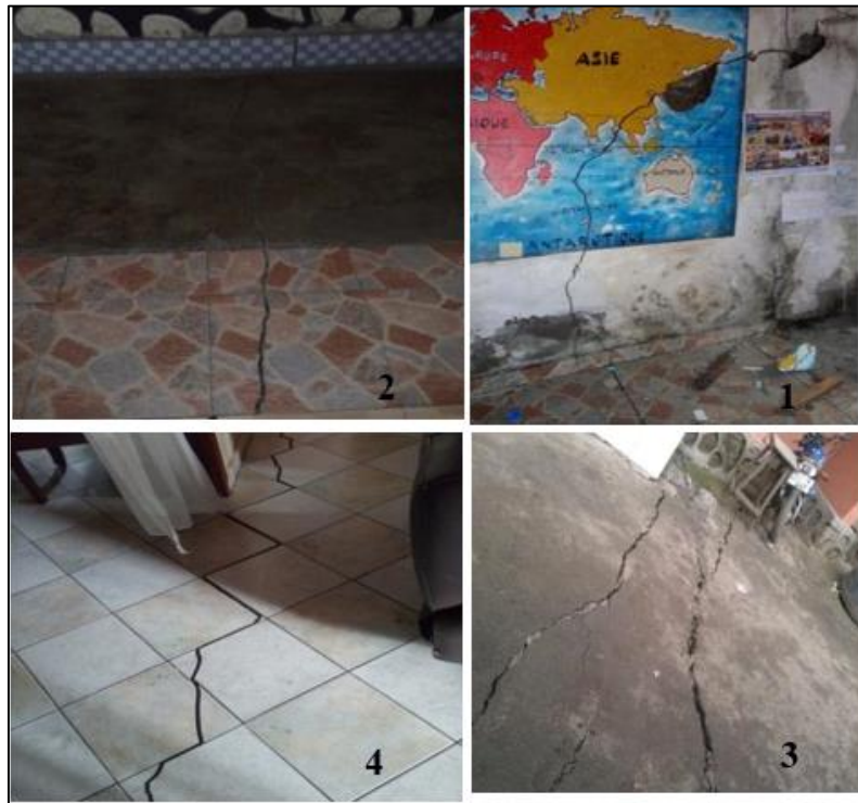
Fig 7: (3, 4) House cracks and (1, 2) Schools
